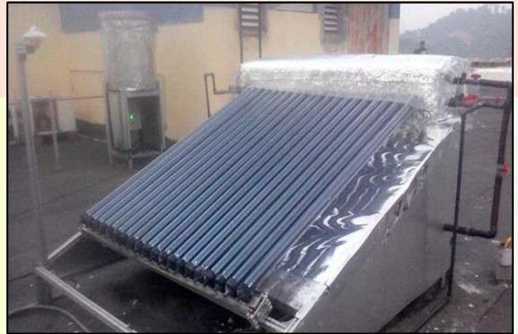
Experimental setup of SWH system and the structure of thermal battery
